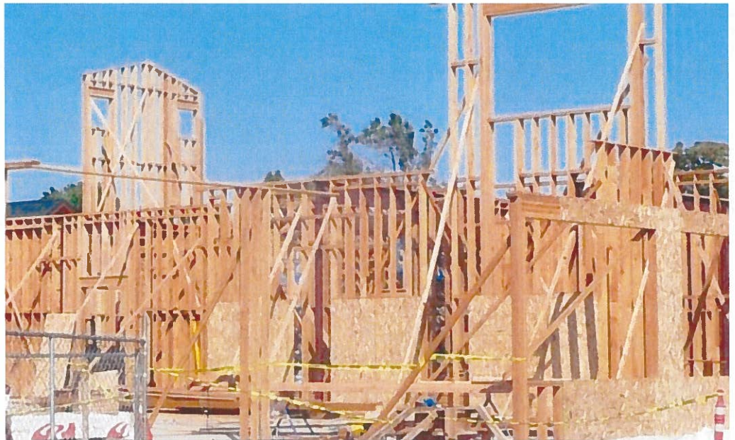
Interior wall and structural steel in Sectors A/B were started in June
