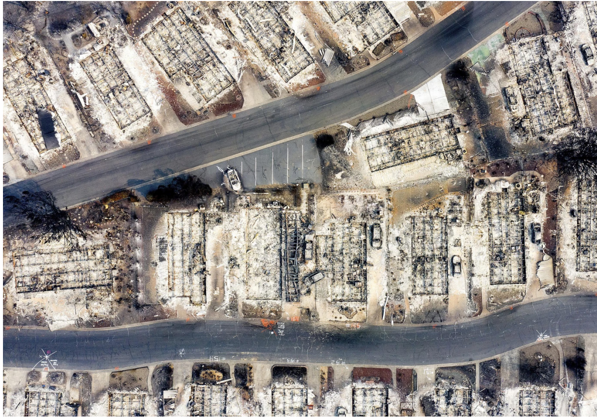
Aerial image showing homes in Phoenix lost in the Almeda Fire in September 2020.
