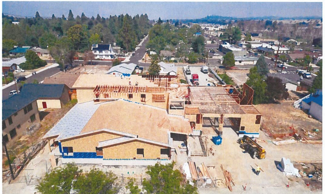
Roof decking at Sector A and trusses at Sector B were substantially complete in August
