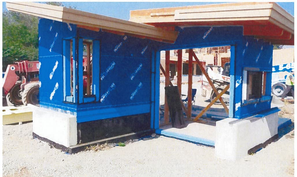
The mockup "Z-Wall" is being used to evaluate installations of windows and weather barrier
