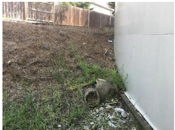
Figure 4: Dirt fill against side of Shop 2 Reservoir
