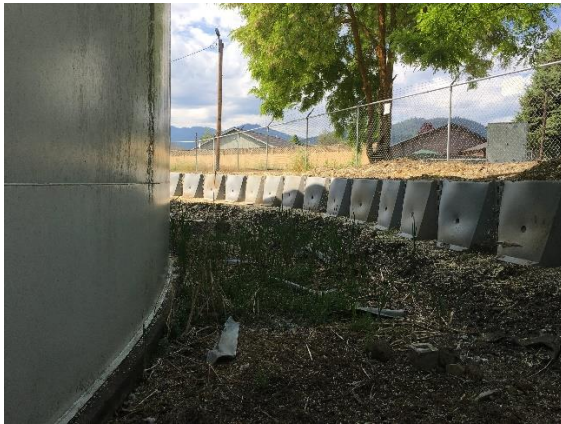
Figure 7: Shop 2 Reservoir Vegetation Growing Against Side of Tank, Poor Drainage
