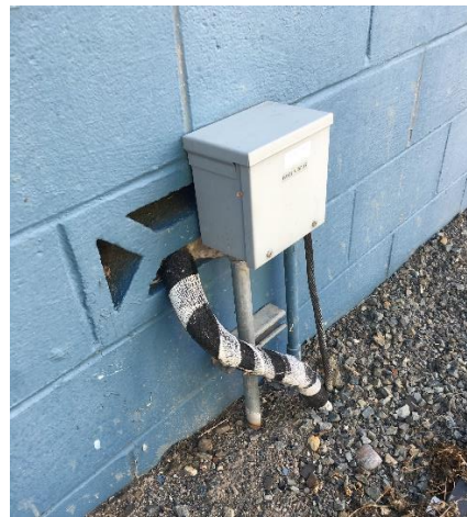
Figure 2: Pressure Transducer Insulated Line Entering Shop Booster Bump Station
