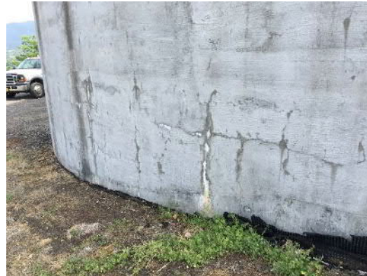
Figure 9: East Side Reservoir Minor Cracking and Efflorescence, Typical
