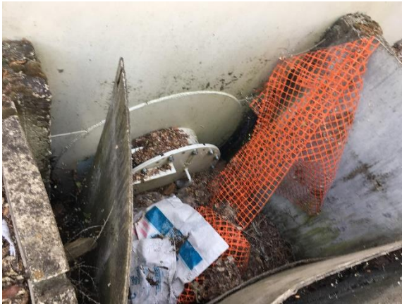
Figure 5: Shop 2 Reservoir Access Hatch not Easily Accessible
