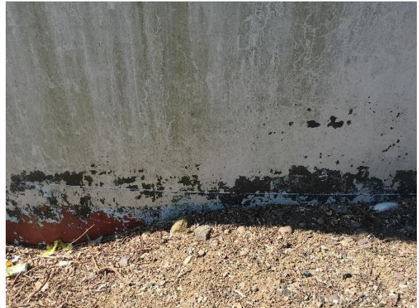
Figure 6: Shop 2 Reservoir Corrosion and Coatings Failure
